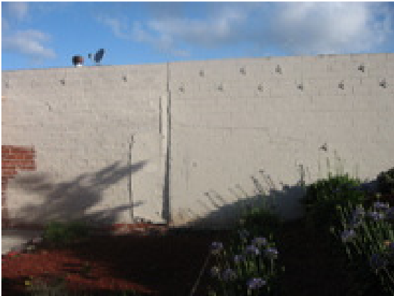
Wall astride the Hayward fault in the East Bay Area
